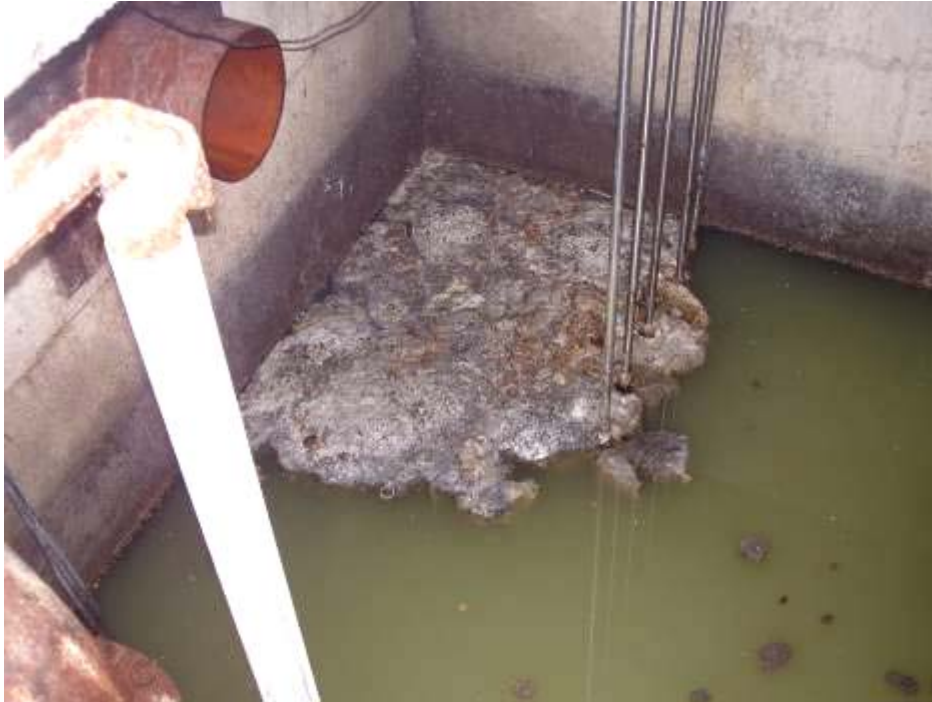
Photograph 8 FOG and debris build up in a ‘dead zone’ caused by a combination of a square tank and cables
